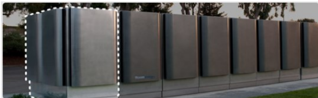
Figure 4: BloomEnergy SOFC system. The dashed region corresponds to the 250 kW e unit [1].
