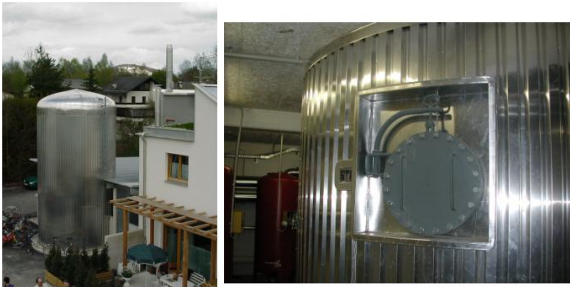
Fig. 11: Water tank for thermal store of solar heat for small district heating (housing estate Gneiss-Moos/Salzburg)
