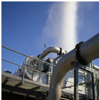
III.1: Cooling towers with vapour formation (product image Company Gohl)
