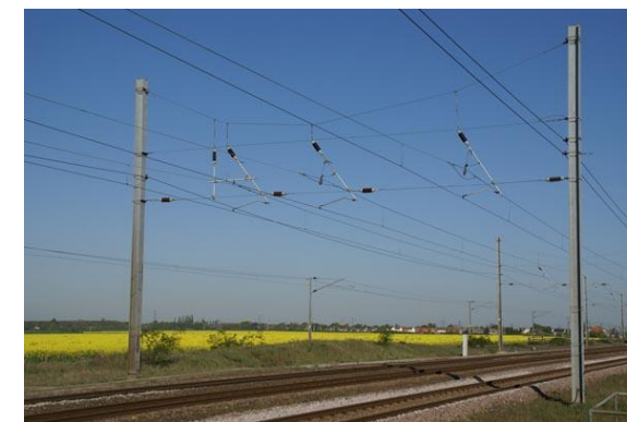
Catenary 1.5 kV DC
