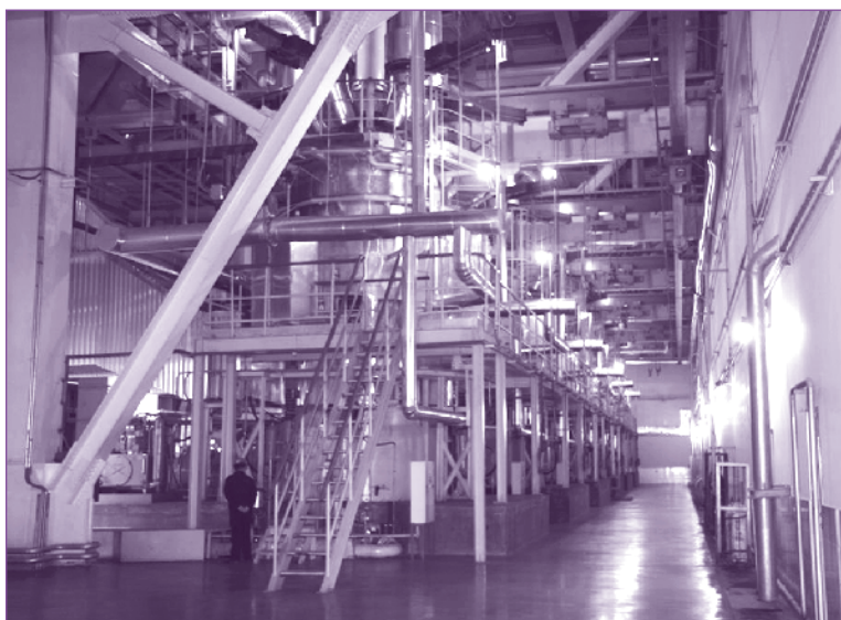
Figure 19 • The mill bay of one of the Wangqu units
