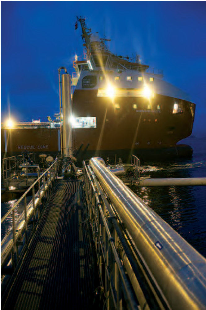
Figure 41: Fixed bunkering lines
