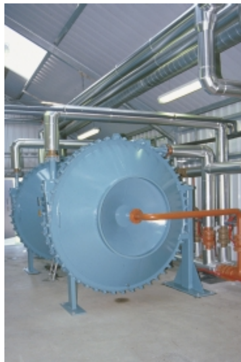
A heat exchanger at the Thorsø plant for heat recovery from digested manure.
