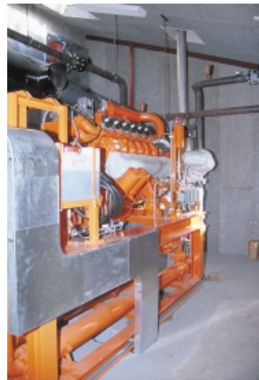
Combined heat and power production facility.
