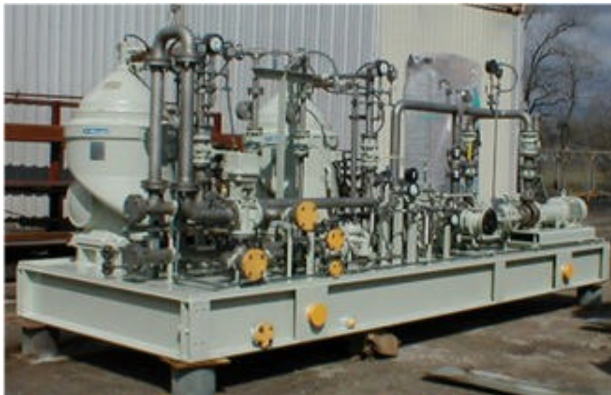
Figure 3-1: Fuel oil treatment plant using AlfaLaval centrifuges [www.marstechusa.com]
